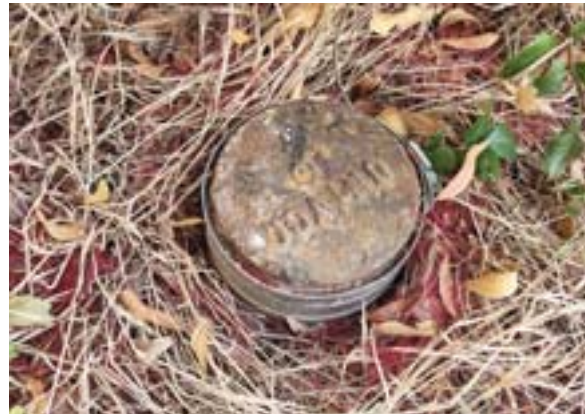
Main Sewer Clean Out
