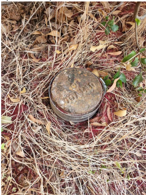
Main Sewer Clean Out Photo Jim Hurley
