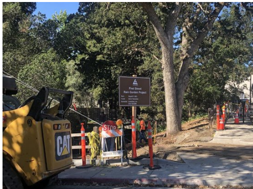
Rain Garden project work on Golden Gate Way in Lafayette. Photo J. Wake
