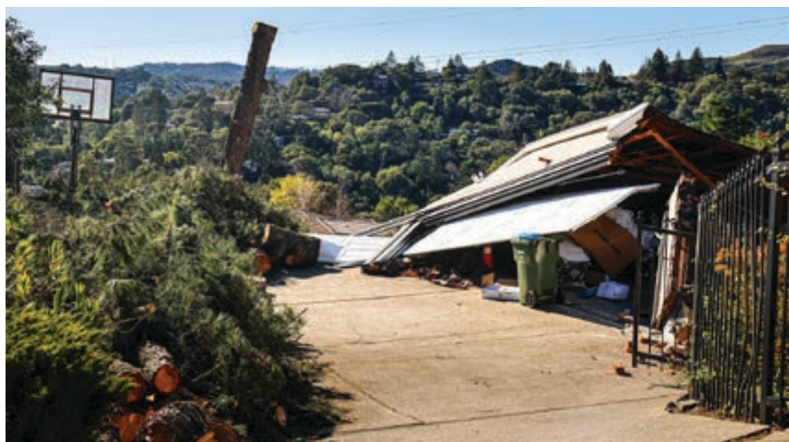
A collapsed garage sits at the end of this driveway on Cedar Lane.
