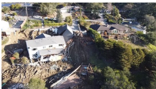
Damaged homes on Cedar Lane in Orinda Photo courtesy city of Orinda
