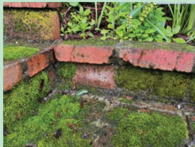
Because of the rainy weather, moss grows on the brick stairs.
