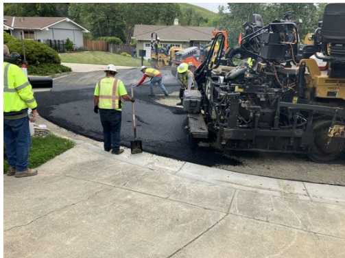
Asphalt repaving on Tia Place in Moraga Photo courtesy Moraga Public Works
