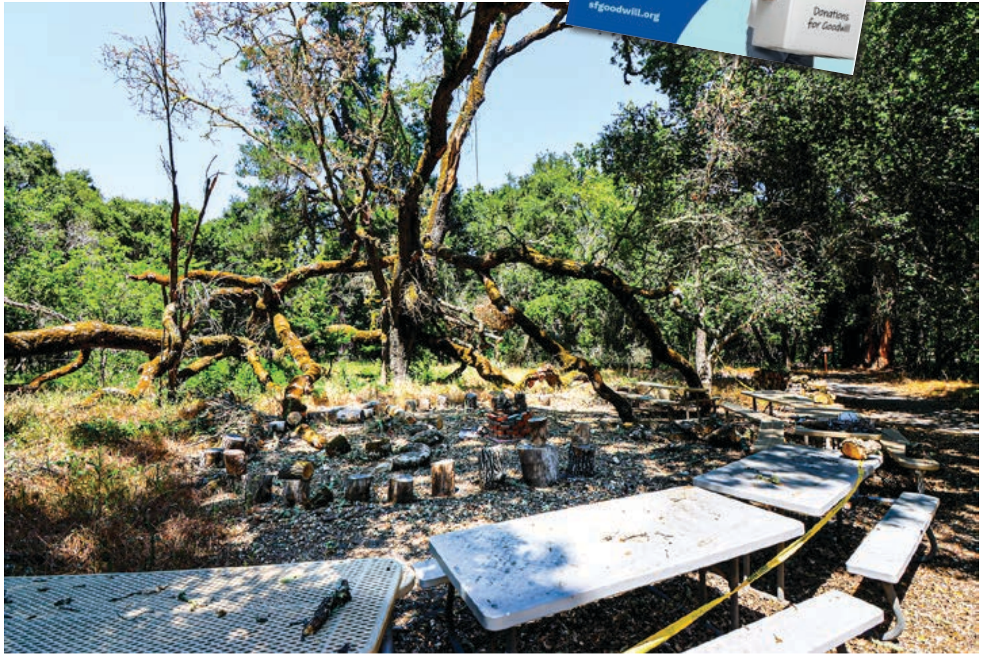
Trees damaged by winter storms pose a safety risk at the Orinda Nature Area.
