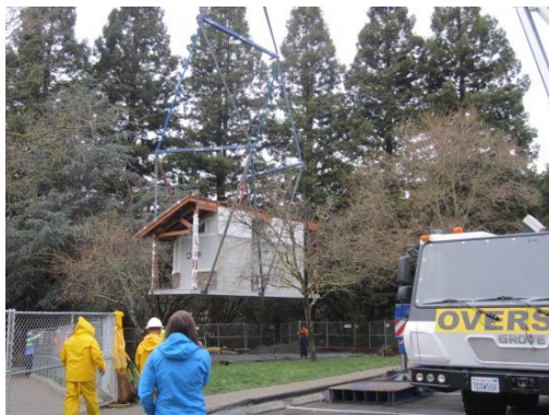
Moraga Commons Park takes delivery of new restroom facility. Photo Vera Kochan
