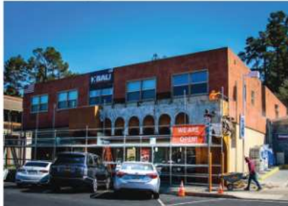
Peets and Nation's get new facades, planned when Nation's moved across the street.
